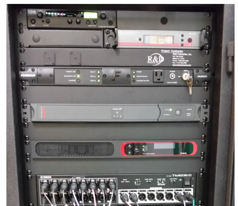
New Equipment Rack
