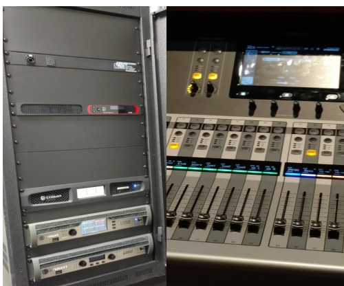
Equipment Rack & New Digital Mixer
